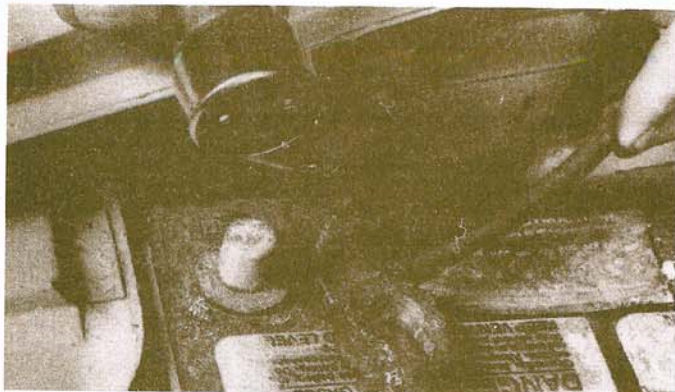
8.7c Regardless of the type of tool used on the battery posts, a clean, shiny surface should be the result
